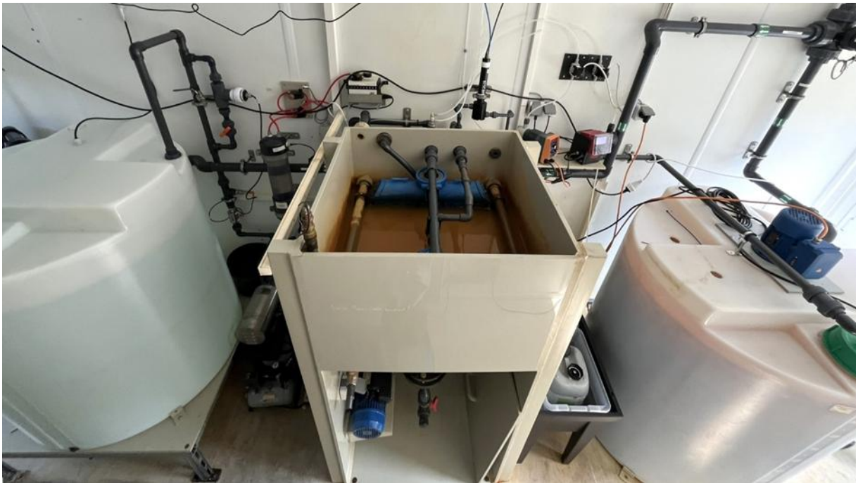
Figure 1: Pilot test with ceramic membrane module submerged in filtration tank (middle), SFBW tank (right) and filtrate tank (left) at waterworks of HAMBURG WASSER
